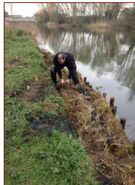
Figure 3: The trial section of pre-vegetated coil rolls being installed on the River Nene in Peterborough
