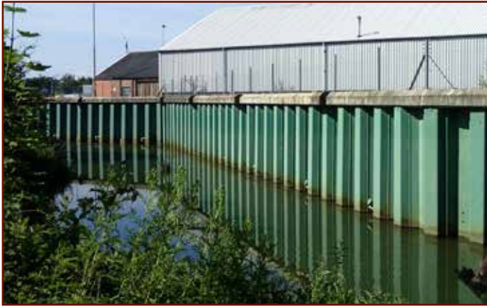
Figure 2: the vertical sheet-piling on the River Nene's Brampton Branch immediately downstream of West Bridge. The piling is unsightly and provides almost no habitat. Our proposed vegetated coir rolls will help to disguise the piling and will provide much-needed habitat.
